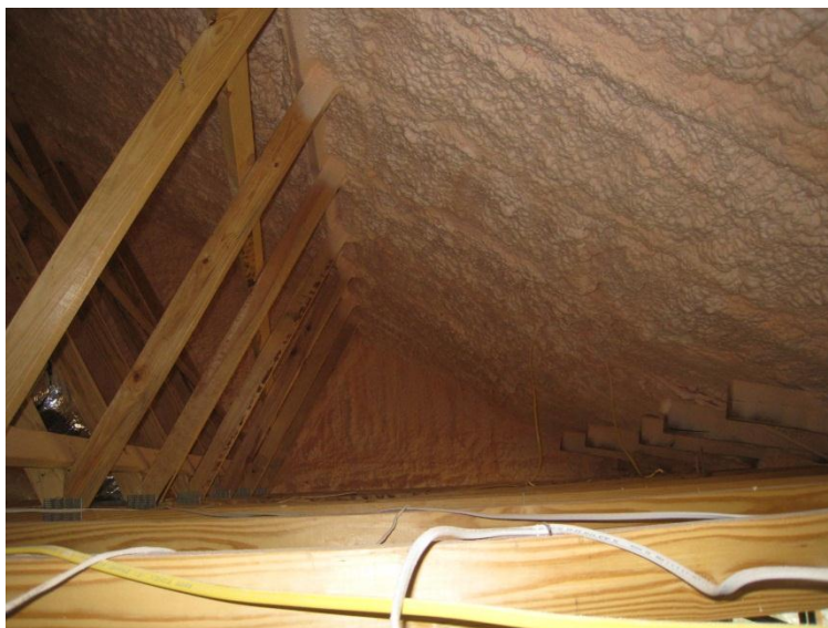
Figure 6 - Spray Foam in an Attic
